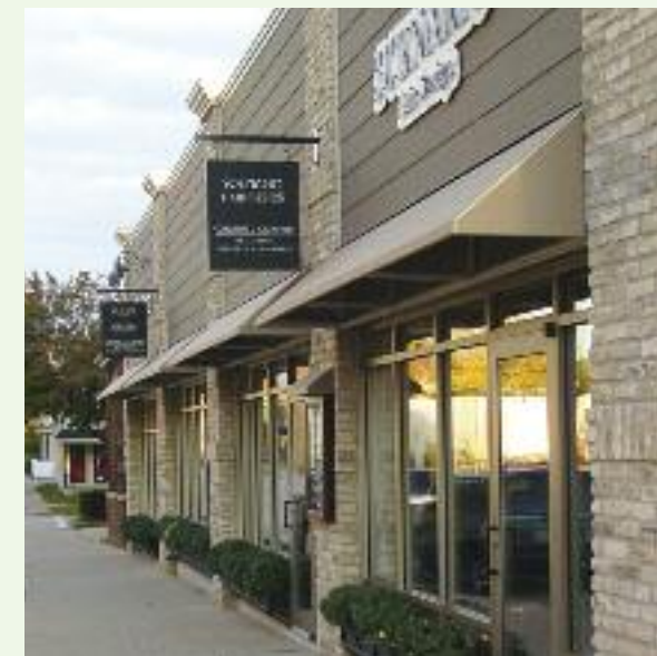
SCHRAMM PROPERTIES 2317-2323 E. CAPITOL DR. Improvements include new windows, blade signs, awnings and brick restoration.
